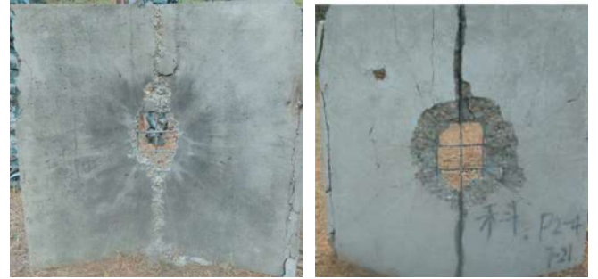
Fig. 4. Slab 11 after explosion, (a) upper face and (b) bottom face [31].
